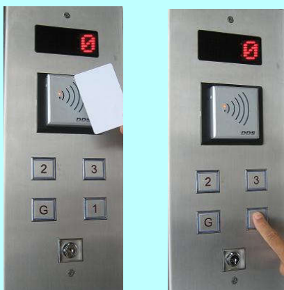
Access Control located inside Elevator car
