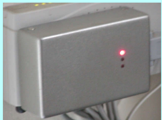
Floor selector located on top of Elevator car/ Machine Room
